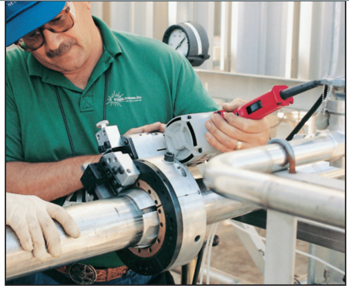
Solution Profile: Piping system contractors performing outage maintenance on thinwall stainless pipe using an electric powered SB clamshell fitted with full support pads. The piping system was part of an auxiliary high purity nitrogen supply line at a semiconductor manufacturing facility. A prefabricated pipe assembly was then orbitally welded in place, without further end prep being required.
