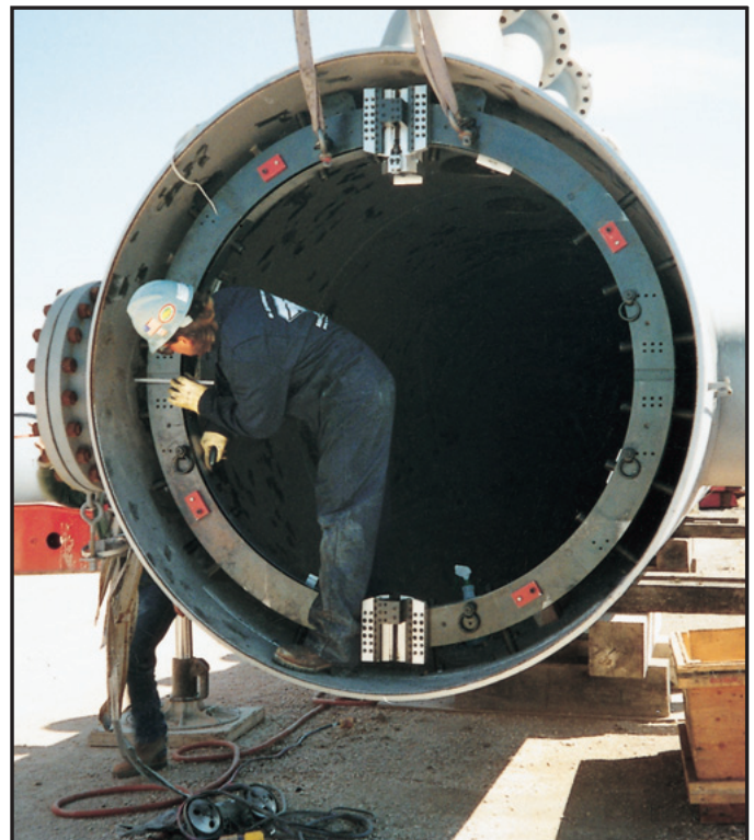
Solution Profile: The versatility of the 600 Series RBL is demonstrated by this Model 660RBL being used in an I.D. mounted role with its mounting screws and tool modules turned to cut from the inside out. This is also why it is important to talk with Tri Tool® sales coordinators and special engineering for non-standard solutions to problems.
